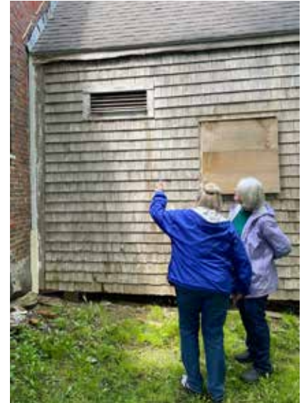
Pittston Historical Society members Rosie Schacht, left, and Louise Kruk, right, examine the joint where the wooden latrine addition is separating from the main brick building.
