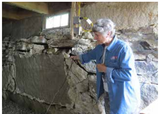
Ingrid Grenon, president of the Vienna Historical Society, indicates where repairs have been made to the foundation of the Milton Bradley birthplace.
